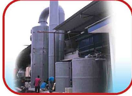
● Online Chlorination System For Glove Industry In Malaysia
