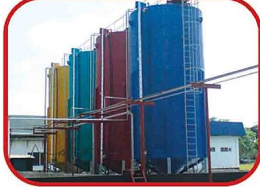
● 4 x 100m 3 FRP Storage Tanks For Palm Oil Industry
